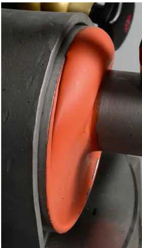
Figure 3. Displacement of the pipeline in lateral direction (perpendicular to the longitudinal direction); the displacement in relation to the transit wall is one sixth of the difference in diameter between the pipe and the transit wall.
